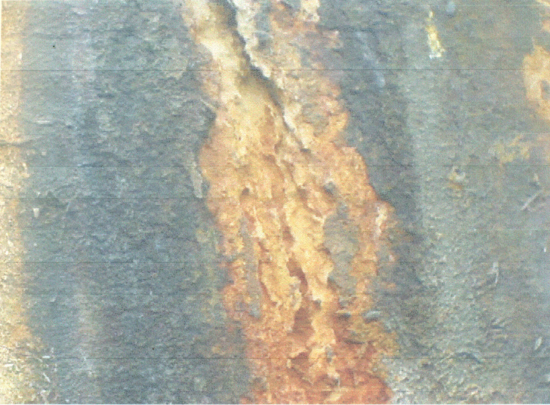
Plate 2.1: Concrete Cracking due to Rebar Corrosion Products. Picture of a Grilled Concrete Wall of the Simon Building Corridor of the University of Manchester
